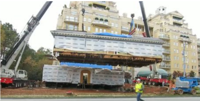
Workers prepare the two sections of the Randolph-Lucas House for relocation. Credit: Buckhead Heritage Society/Terry Kearns
